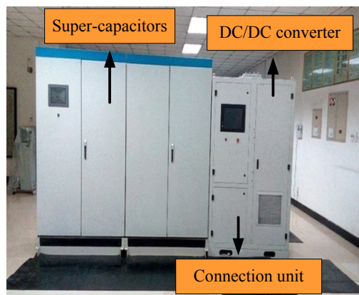
Figure 7. Super-capacitor ESS installed in traction substation.
