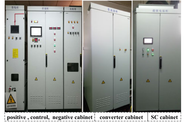
Fig. 15. Photos of the 1-MW ESD installed in LIYUAN substation.
